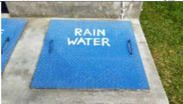
15(h) Rainwater Reservoir in Faculty of Engineering
