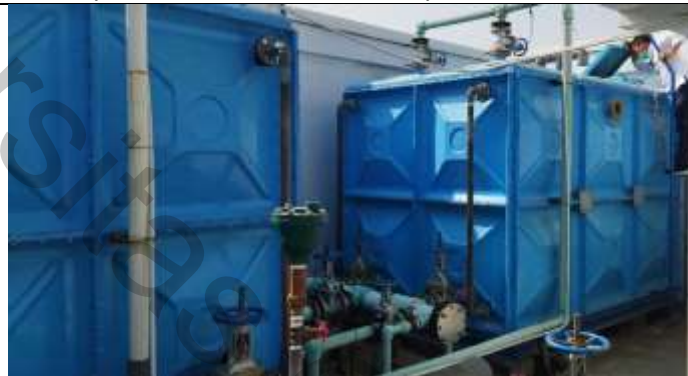
Figure 3 Greywater installation at Faculty of Economics and Business
