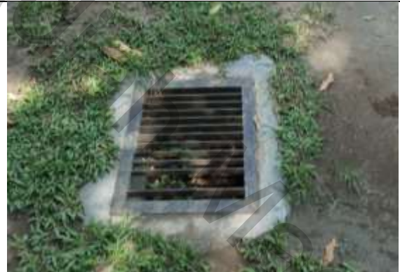
15(c) Infiltration Well in Faculty of Cultural Science
