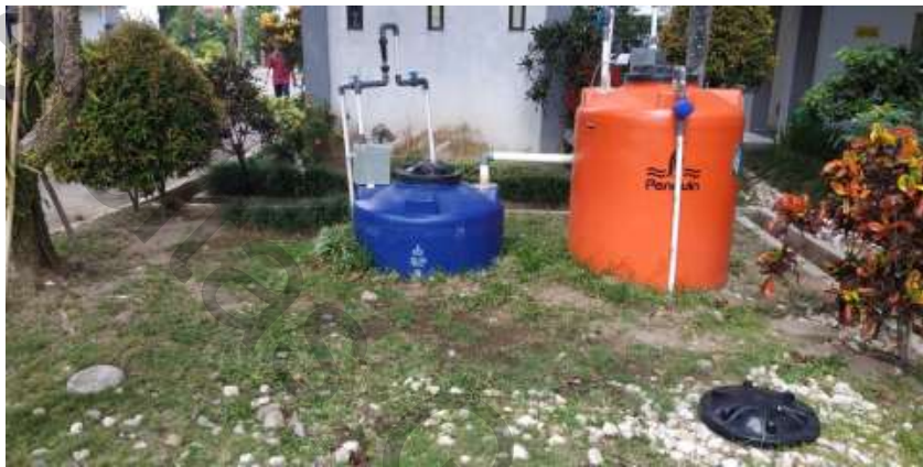
15(d) Underground collector tank at UGM Residence
