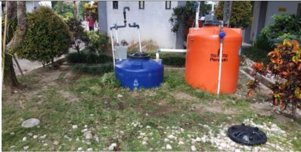
Figure 6 Underground collector tank at UGM Residence
