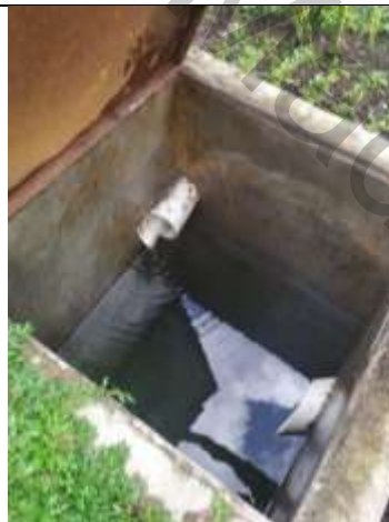
15(k) Rainwater Reservoir in Faculty of Engineering
