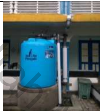
15(i) Rainwater Reservoir in UGM Residence
