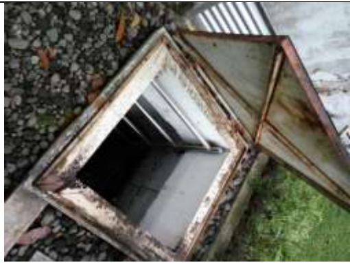
15(g) Rainwater Reservoir in Library of UGM
