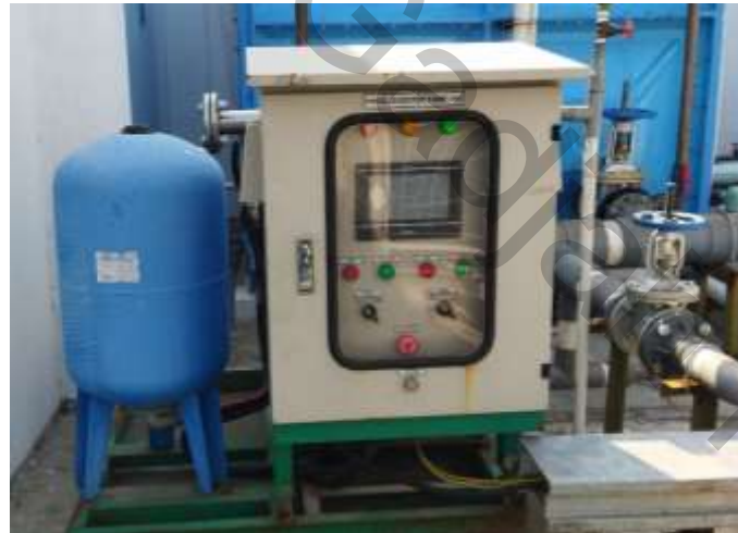
Figure 4 Greywater installation at Faculty of Engineering (SGLC building)
