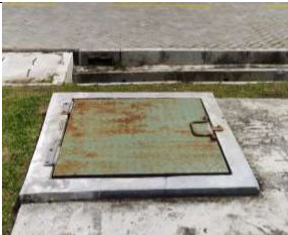
15(j) Rainwater Reservoir in Field Research Center
