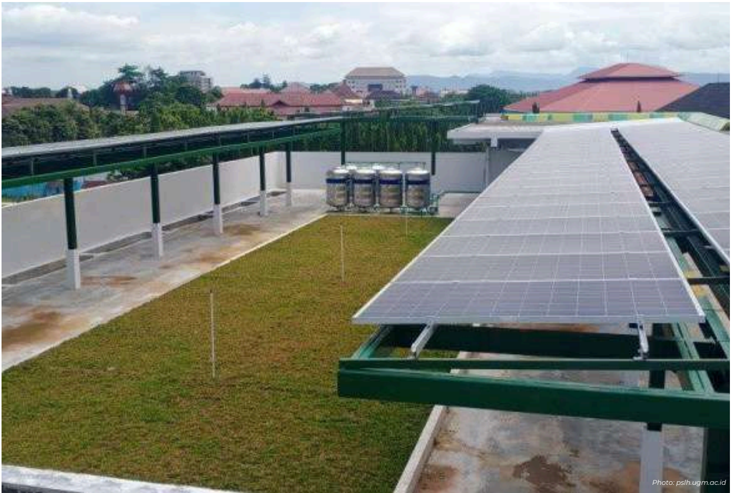
Solar panel system in Center for Environmental Studies among many of newly installed UGM
