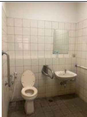
Figure 23 Toilet for Disabled People (People with Special Needs) at Faculty of Agrotechnology
