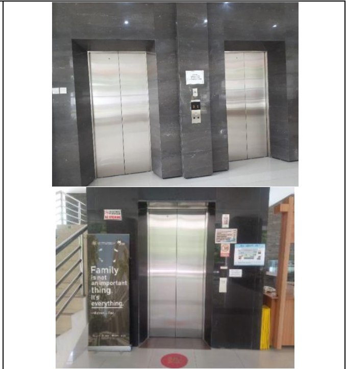
Figure 29 Lift for Disabled People (People with Special Needs) at Faculty of Agriculture and Political Sciences
